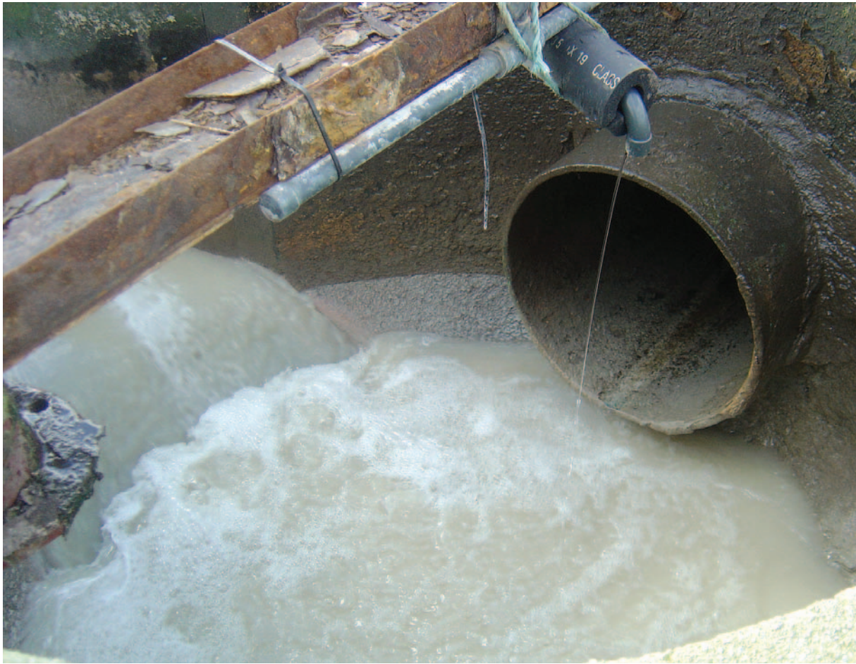
FIGURE 1 Coagulant dosing into an influent wastewater channel
